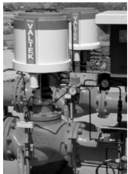
(Right) A liquid nitrogen loading facility in Australia uses two Mark Ones for its emergency fire water system.
