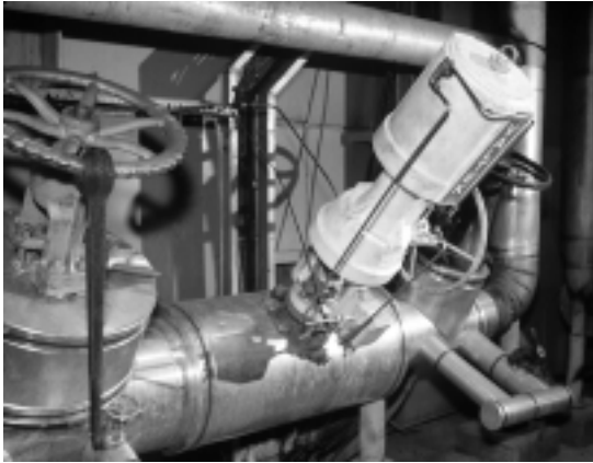
A four-inch Mark One with side-mounted handwheel operates in a boiler feedwater system at a pulp plant.
