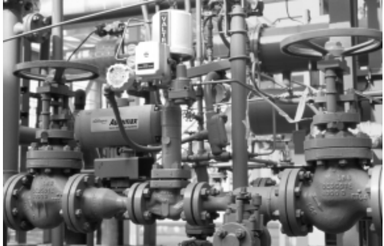
This two-inch Gaurdian II operates in a chemical plant.
